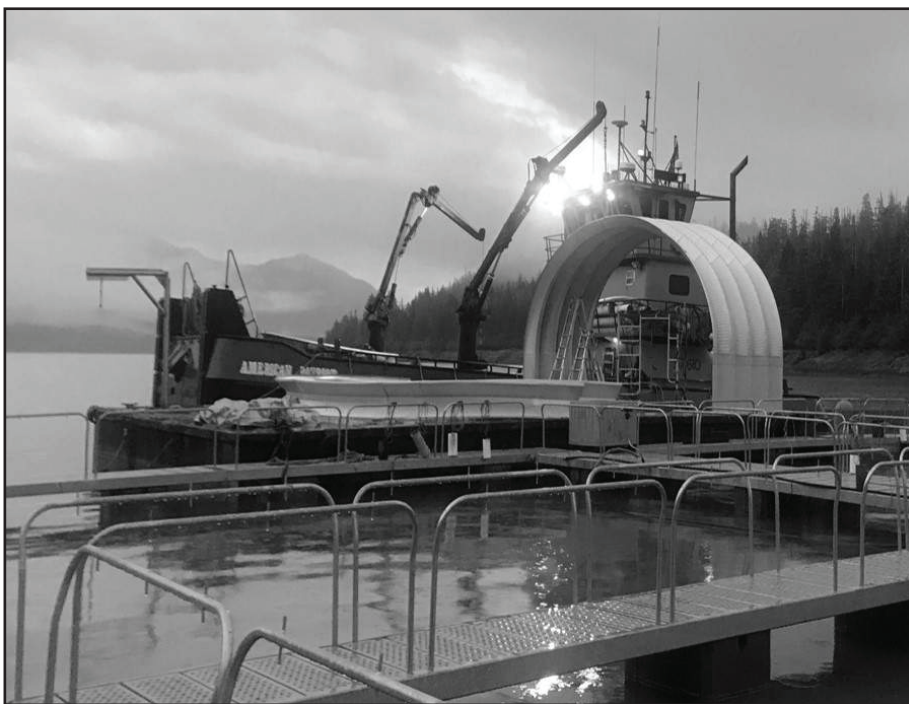
Thomas Bay added a feed float this summer. Construction was completed in a few days by NSRAA staff with the assistance of the American Patriot.
