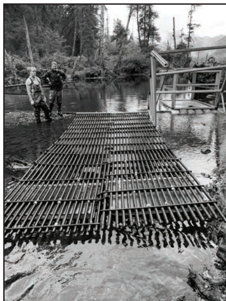
The Salmon Lake crew, led by Ben Adams, completely rebuilt the Salmon Lake weir this summer. Alyssa and Annie work on putting the weir together.
