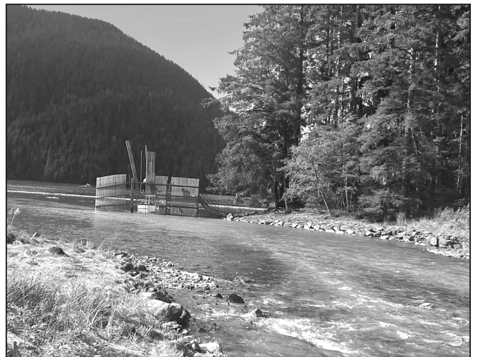
Lower weir in Medvejie Creek after flood damage
