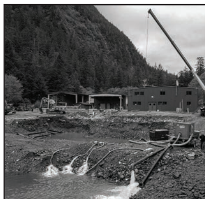
Much of the work had to be done during negative tides. Pumps were needed to dewater the site during base preparation.
