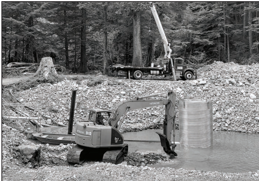
A new water intake is installed at Medvejie. The thirty-foot-deep structure was designed in an attempt to improve water quality and to reduce pumping at the hatchery.
