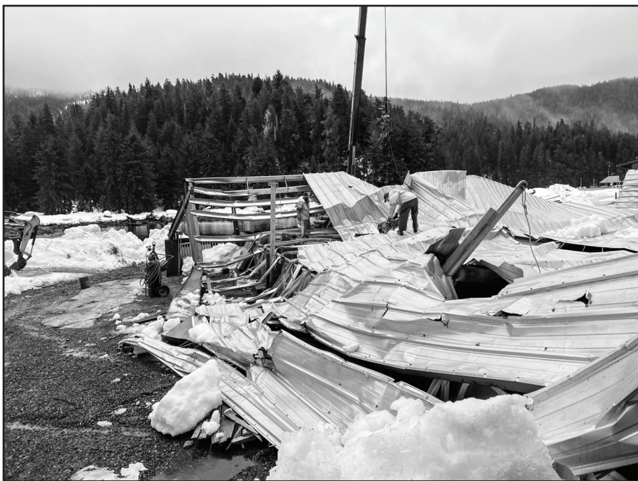
One area of the Hidden Falls roof collapse that happened early this year
